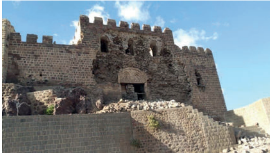
Figure 5. (b) Al Quahira Castle gate house, Yemen, after collapse, February 2024. Courtesy of Heritage for Peace (Isber Sabine).
