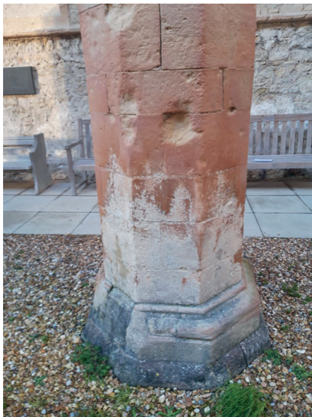
Figure 3. Combined bomb blast, fire, and salt weathering damage on a pillar of the Royal Garrison Church, Portsmouth, UK. Photograph by the author.
