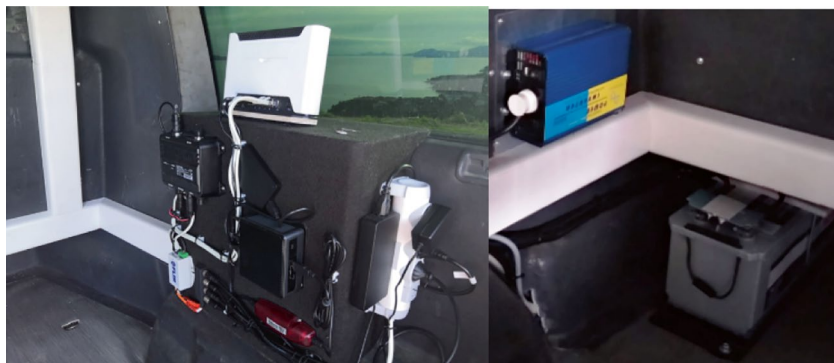
Fig. 30.4 Photographs of the telecommunication equipment and the power system battery installed in the rear cabin of the HCG patrol van
