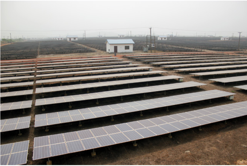
FIGURE 3.3. BXC solar power station, Winneba, Ghana, 2020. Photo by the author.
